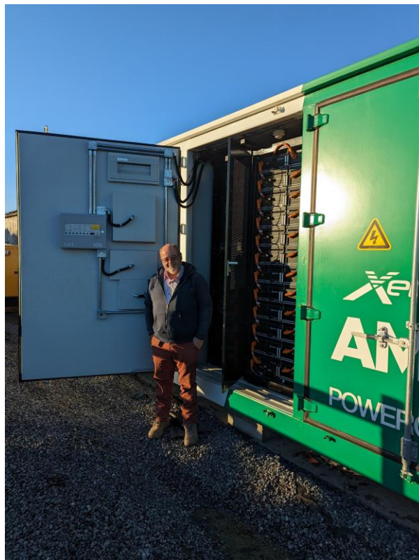
3 - Geraint and the battery storage at Bargoed Farm
